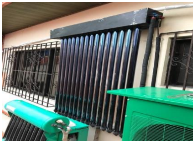
Figure 1: Evacuated tubes solar collector
