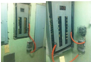
Figure 7. (Left) Kilowatt-hour meter was used for the lights and fans (Right) Two kilowatt hours attached into the connection
