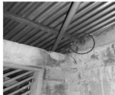
Figure 3. Broken Steel Purlins of COPE Housing Design Variant brought by rusting of members due to monsoon rains (encircled)
