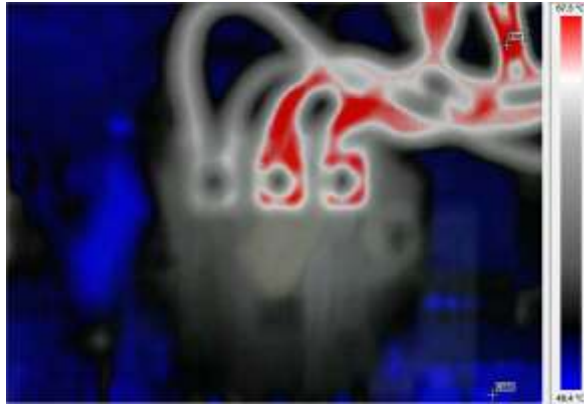
Fig. 11. Unbalanced lines seen in the contactor similar to Figure 1.
