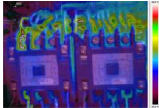
Fig. 4. Similar to contactors and transformers, relays should have no resistive terminals causing excessive heat. All terminals should be retightened by the maintenance engineer.
